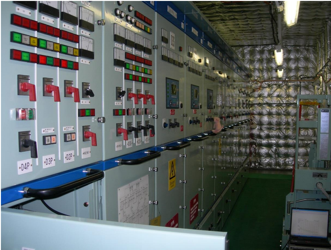
Electrical switchboard in marine environment
